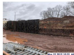
Mar 22 2019 10:22 AM Rebar and form work for south foundation wall, center sector
